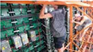
Difficult to maintain, High maintenance costs
